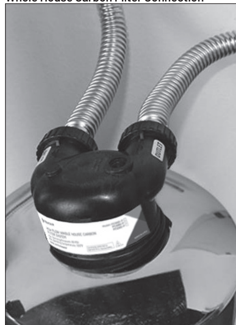
Whole House Carbon Filter Connection
